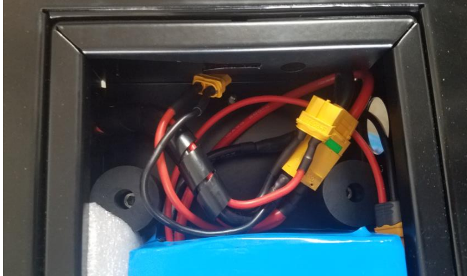
GOOD - cables placed away from door and key latch
