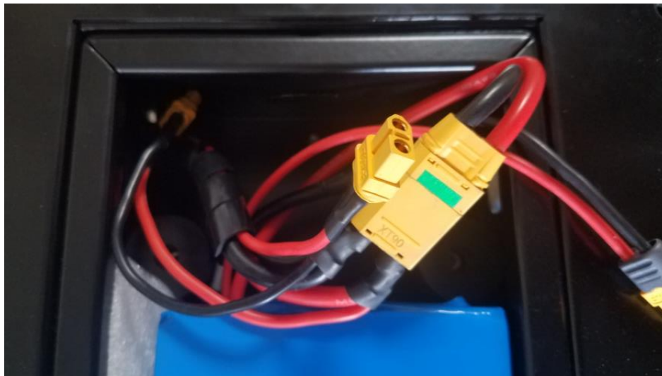
BAD - cables obstruct door closure
