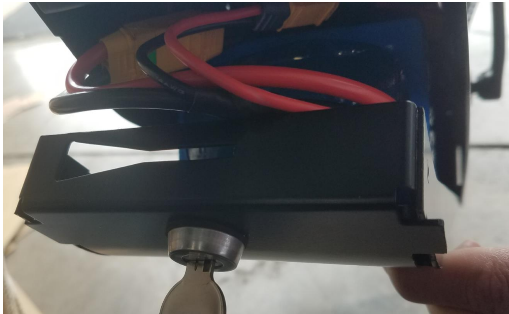
BAD - Cables will be pinched by cover
