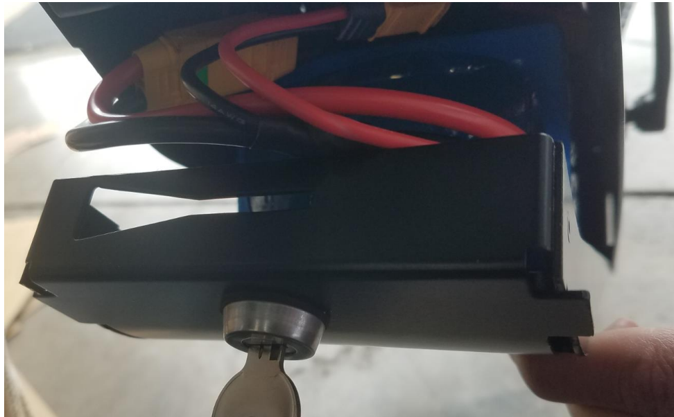
BAD - Cables will be pinched by cover
