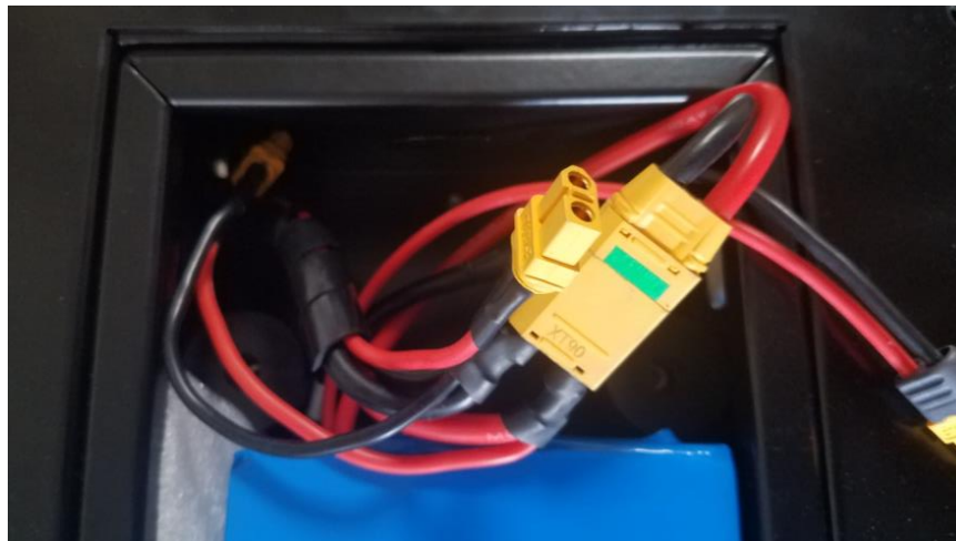
BAD - cables obstruct door closure
