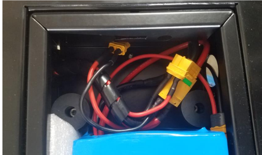
GOOD - cables placed away from door and key latch
