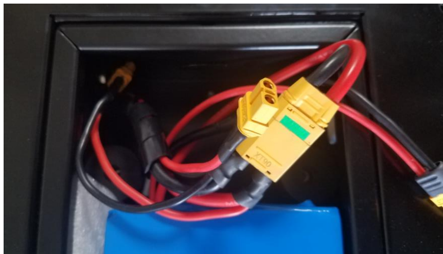
BAD - cables obstruct door closure
